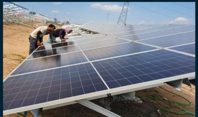
2.4 mw ground mounted on grid EPC on Bhopal M.P.
