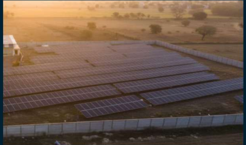
5 mw ground mounted on grid EPC on Bhopal M.P.
