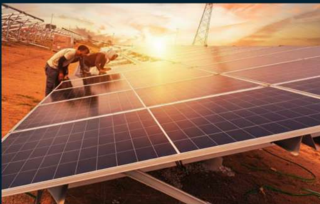
2.4 mw ground mounted on grid EPC on Begamganj M.P.
