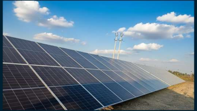
2.4 mw ground mounted on grid EPC on Raisen M.P.
