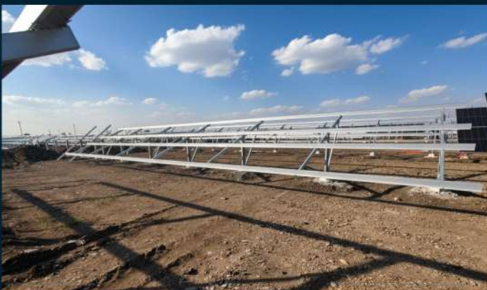
2.2 mw ground mounted on grid EPC on Rajnagar, Dist.-Chhattarpur M.P.
