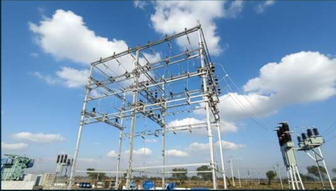
20 mw ground mounted on grid EPC on Guna M.P. (open access)
