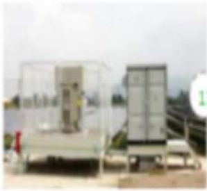
INV Transformer Yard
